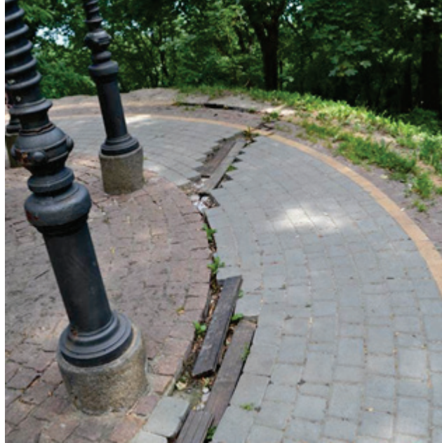
Figure 1 Cracks in the paving around the gazebo caused by the base uneven deformation; the crack opening width exceeds 50 mm.
