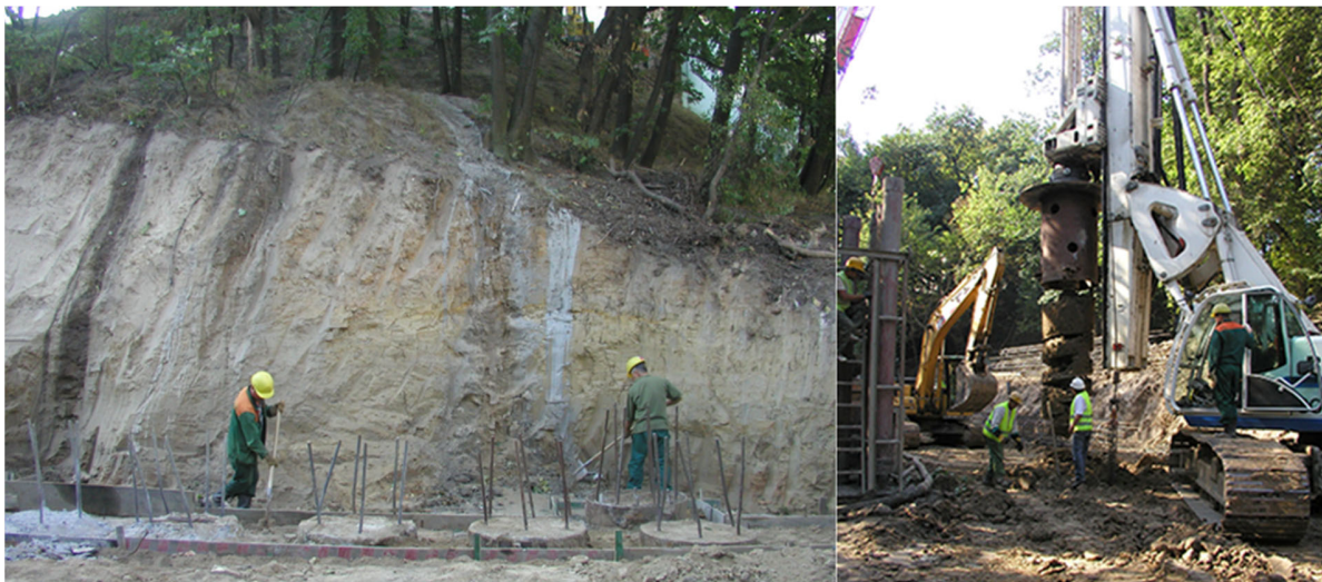
Figure 3 Strengthening the stability of the hill of St. Andrew's Church with the help of bored piles
