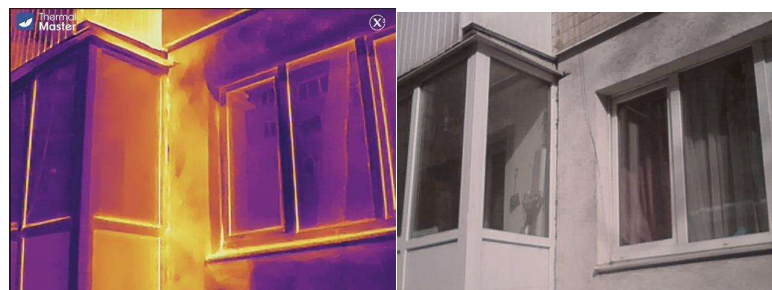
Figure 3. Thermal leakage occurring where panels are joined. Warm colors like orange and yellow indicate higher temperatures; cooler colors like blue and purple indicate lower temperatures. Since these readings were captured on the building exterior during winter, higher temperatures suggest where insulation is poor or where heat could be escaping
